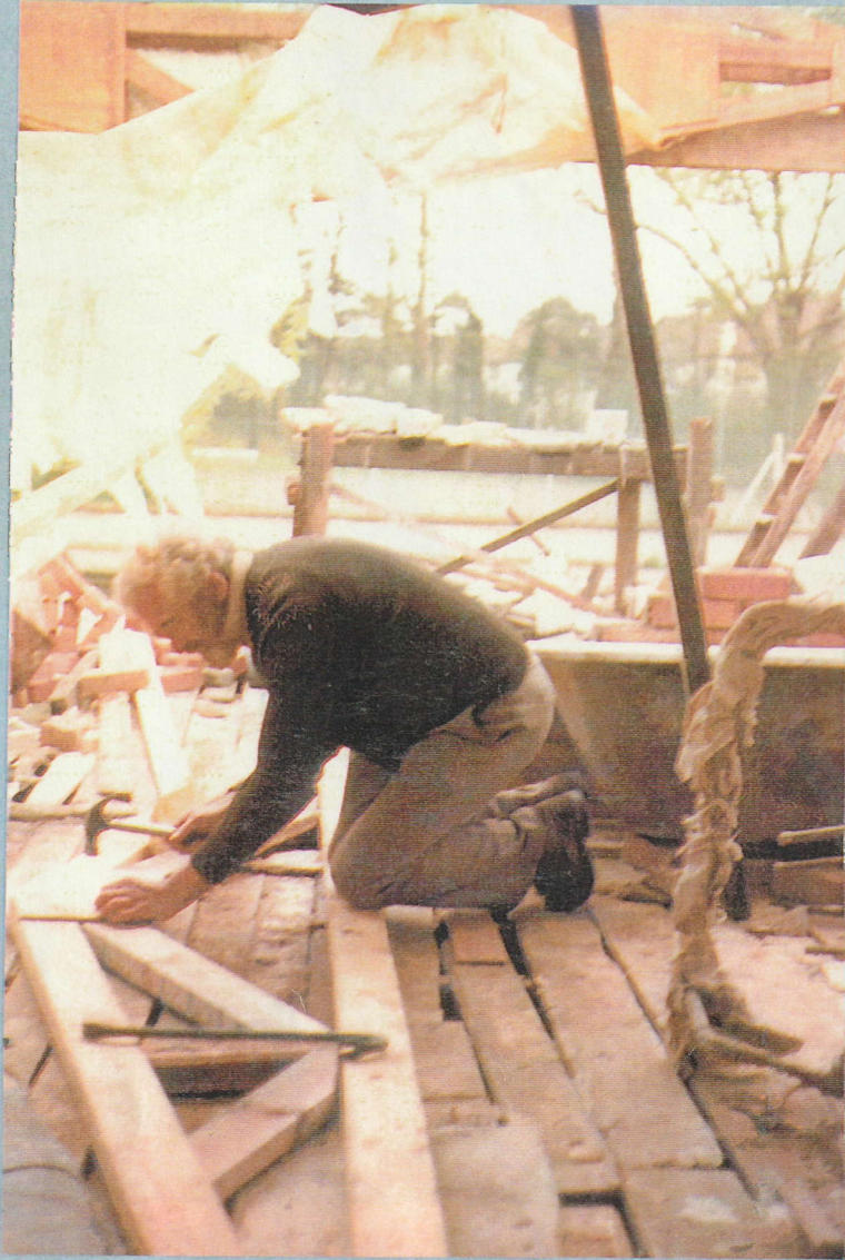
Jack in late 1981 making a roof truss -the Building Inspectors put him through it... 17 of these at 2' intervals
